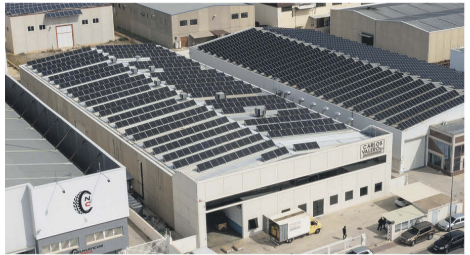
• Carlos Valero, S.L. / 108 kWp
